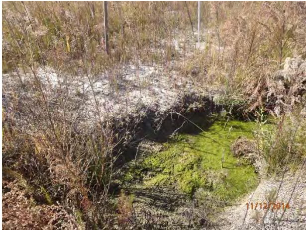
SP3 Minor LB Erosion at STA 25+70
