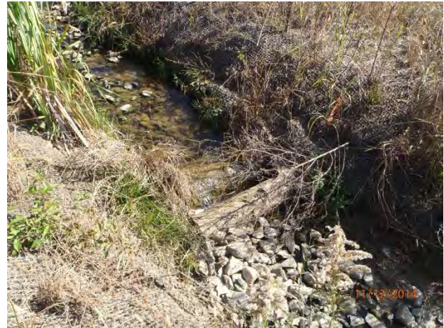
SP4 Minor Bed Erosion at Sta 47+15 - 47+45
