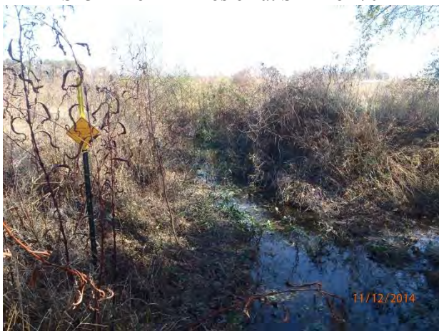
SP5 Minor RB Erosion at Sta 5+60
