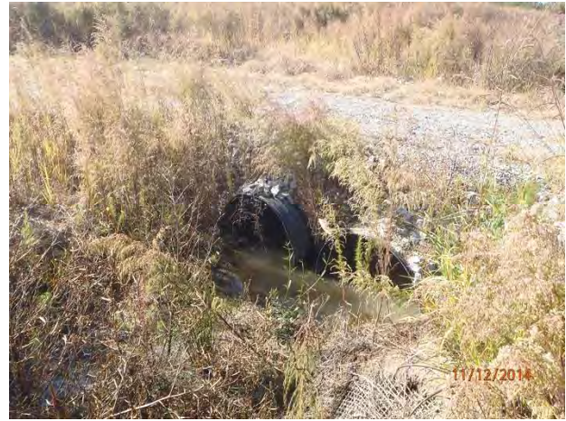
SP2 Minor RB Erosion at STA 21+50
