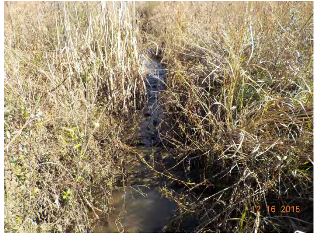
SP2 Minor Bed Erosion at Sta 47+15 - 47+45.
