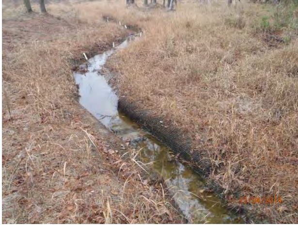
SPA1- Loose grade control toe log structure - Reach 2 @ Sta 3+25
