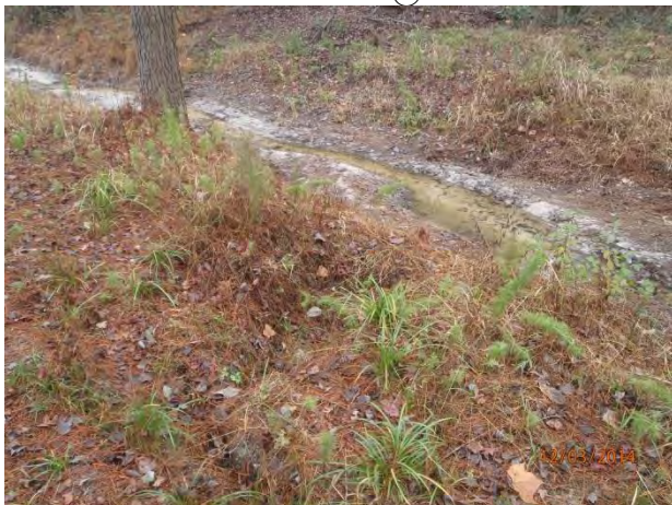
SPA5- Minor left bank erosion – Reach 3C @ Sta 60+00 and 61+00
