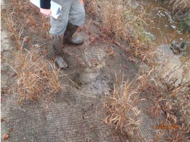
SPA7- Minor right bank erosion- Reach 5A @ Sta 14+00
