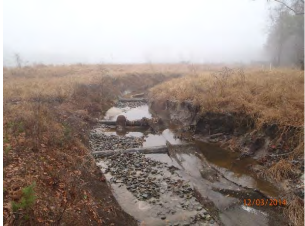
SPA8- Failed grade control structures, bed/bank erosion- Reach 5A @ Sta 16+50- 19+50
