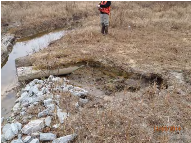
SPA3- Left bank erosion behind flow diversion structure - Reach 3b @ Sta 37+22
