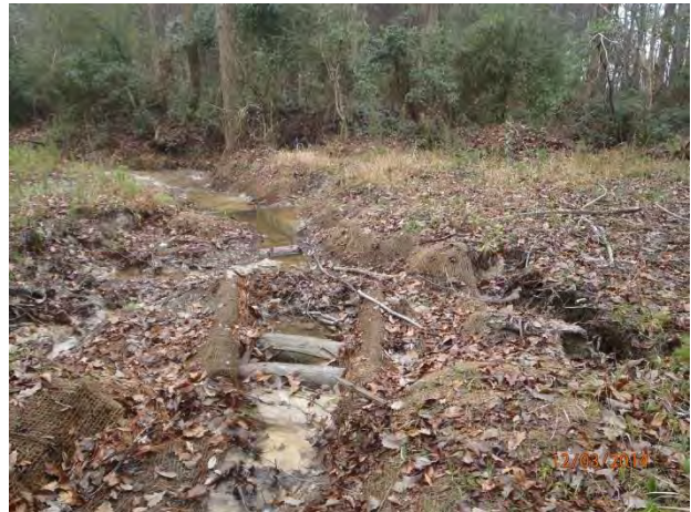
SPA4- Failed grade control structures- Reach 3B @ Sta 57+30 – 57+80
