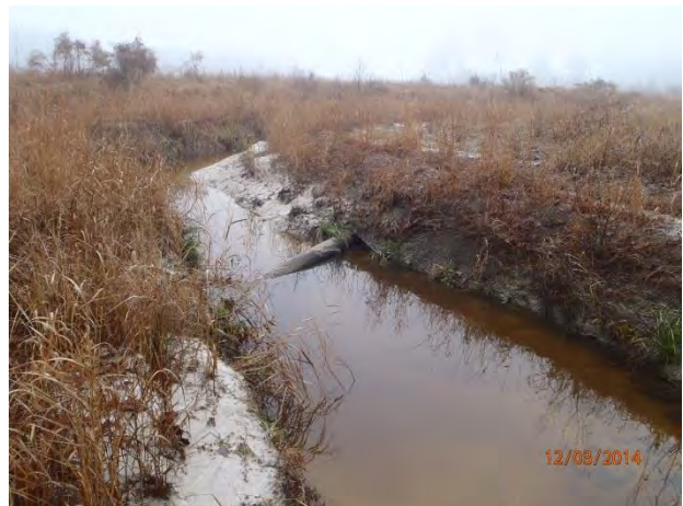
SPA6- Failed grade control structures and bank erosion- Reach 5A @ Sta 13+25- Sta 16+50
