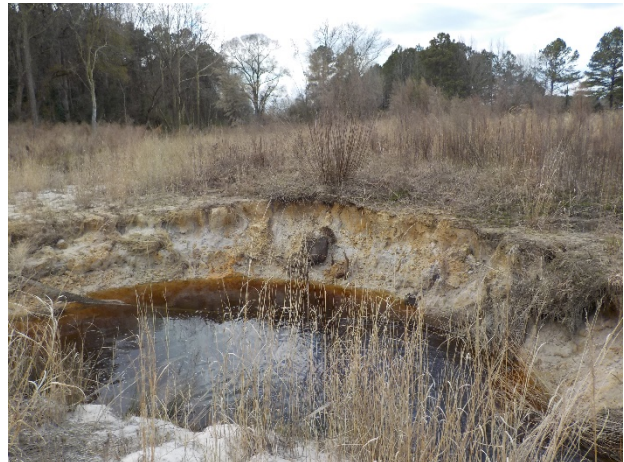
SPA5- Right bank erosion- Reach 5A @ Sta 14+00
