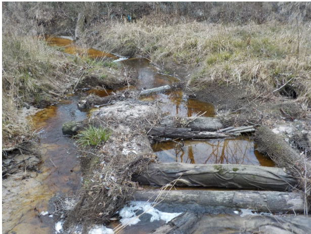
SPA3- Failed grade control structures- Reach 3B @ Sta 57+30 – 57+80
