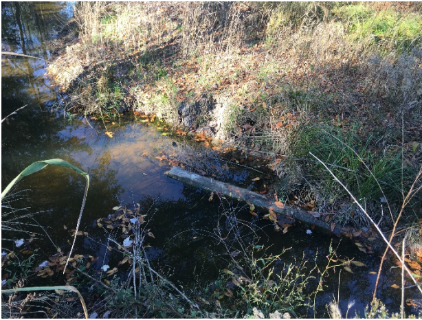
MY4 – SPA1 – Right Bank Erosion on Reach 5A at Sta. 19+50
