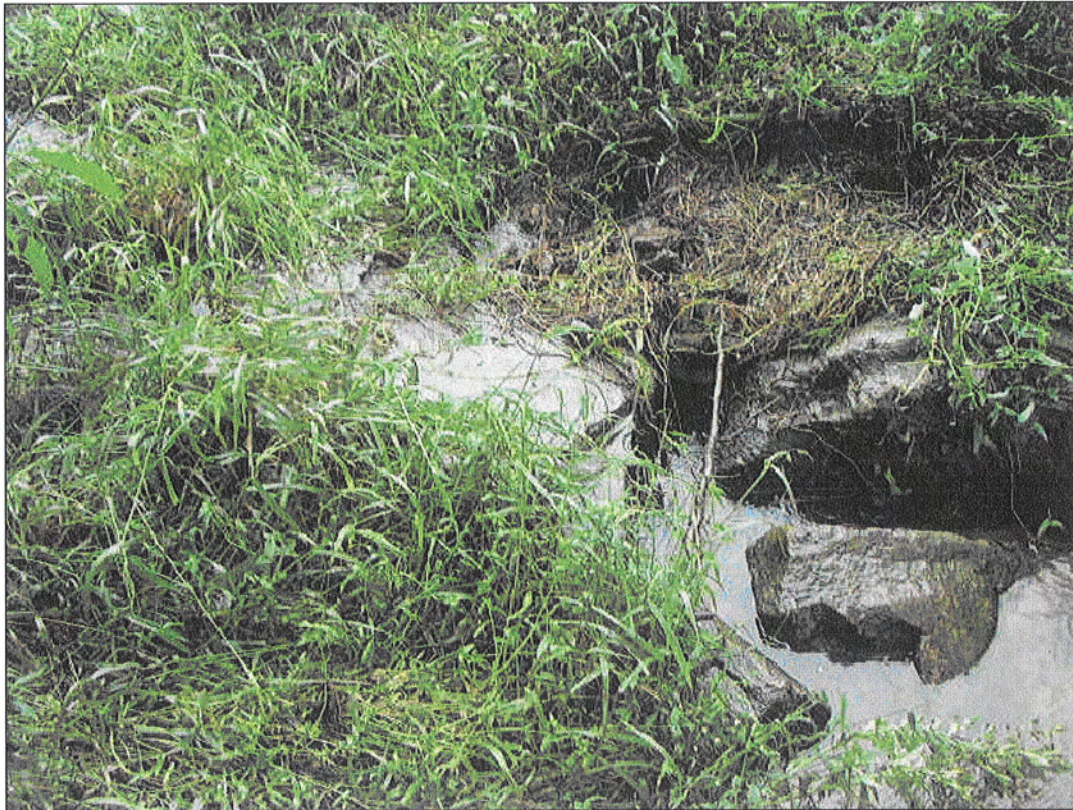
STREAM PROBLEM AREA 3: PIPING AT STRUCTURE LOCATED AT STATION 34+67.
