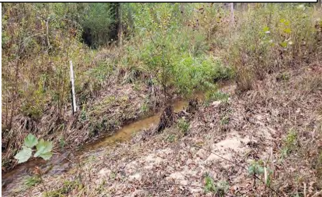
Photo 3: Wrack, sediment, and laid-back vegetation in the floodplain of Neighbors Branch
