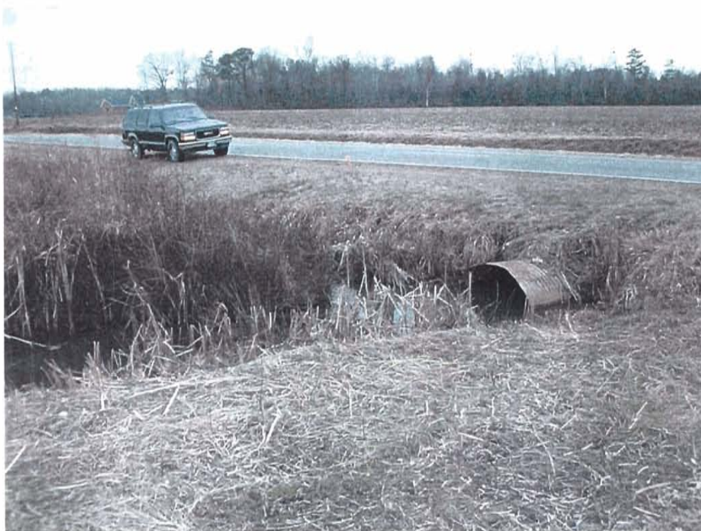
Figure A4. Road culvert under British Road (SR 1803) at end of project site
