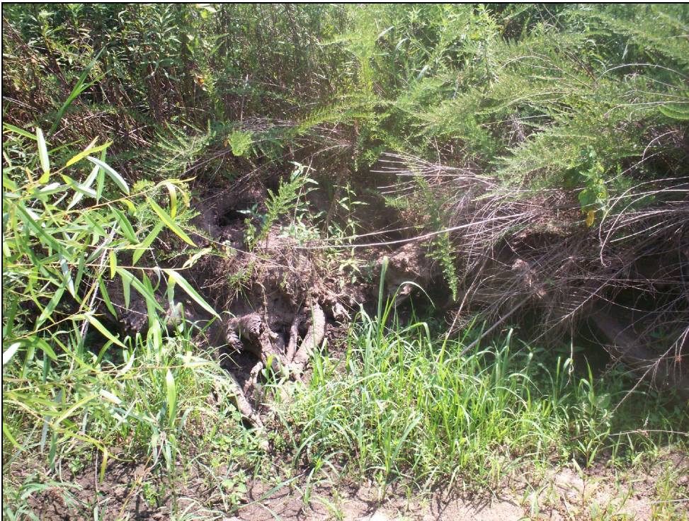
Photo 10 Station 13+75 Reach 2 right bank. Root wad.
