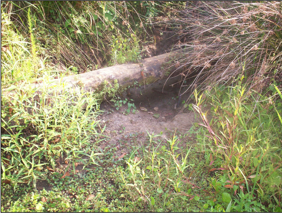
Photo 1 Station 28+75 Reach 1 upstream. Problem area-undercut log vane.
