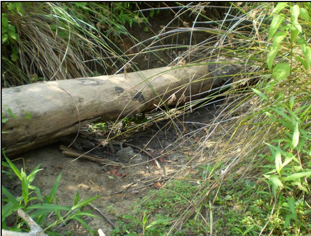
Log vane @ station 29+00 (Reach 1), channel is washing under the structure.
