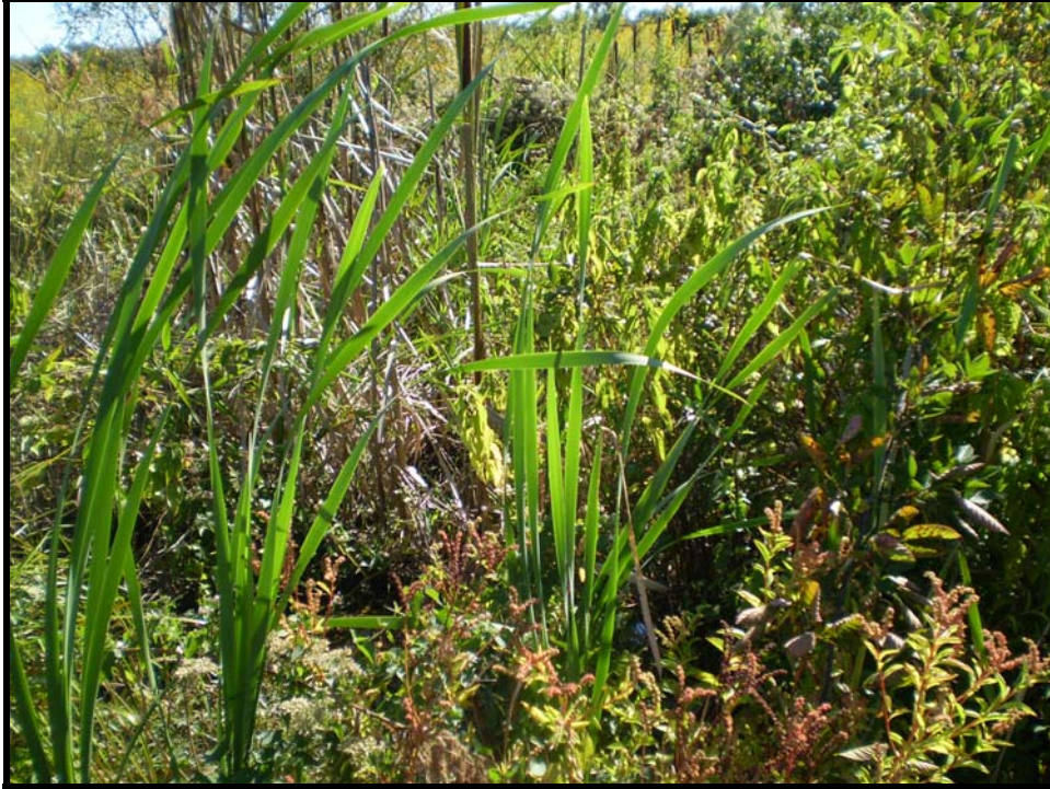
Reach 5 – Heavy vegetation in channel throughout reach, restricting flow (PA5)
