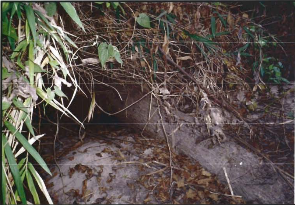
SPA 1. Undercutting at log vane (approx. 1') STA 20+40.
