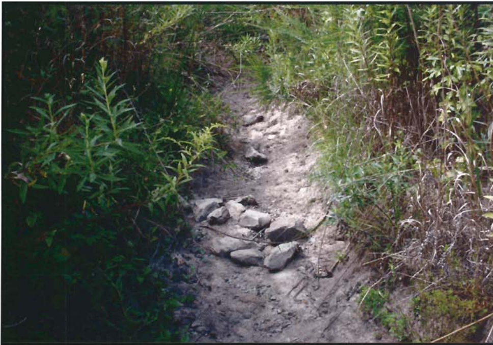
SPA 4. Rock cross vane failure at STA 52+00.
