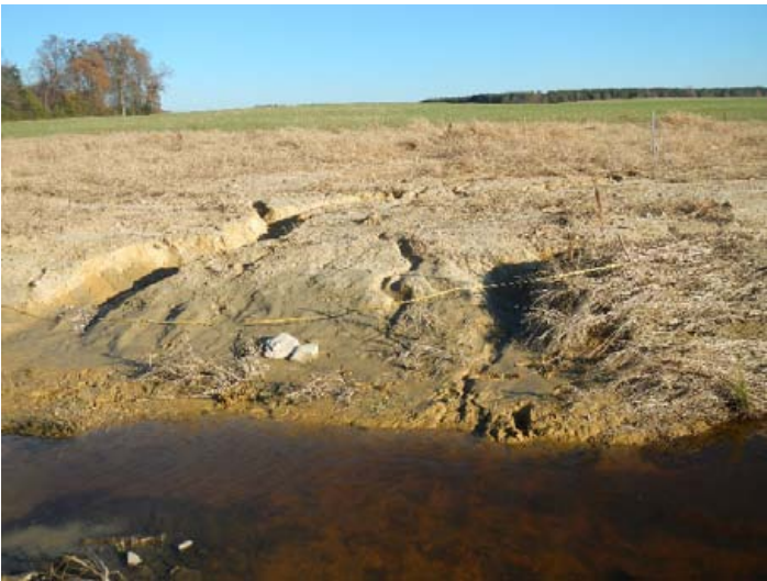
AOC-3: Rill erosion Norkett Branch Reach 1 right bank, 12-1-2014
