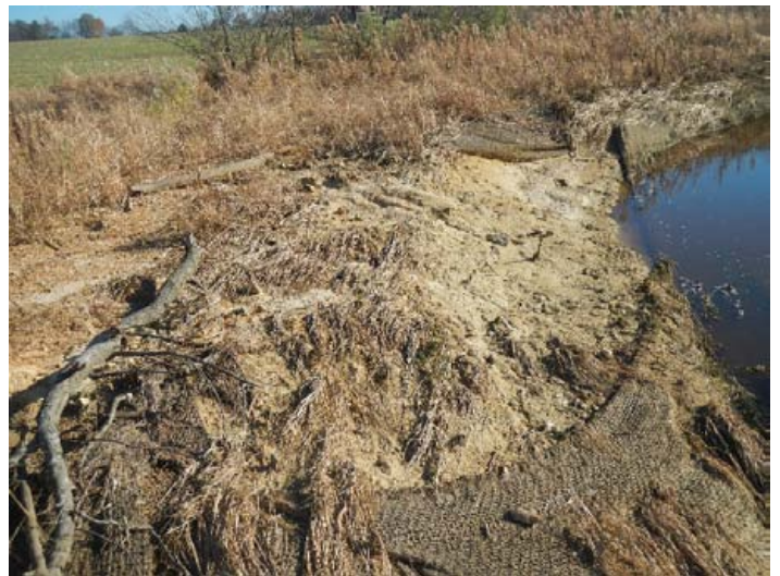
AOC-6: Loose mat Norkett Branch Reach 1 right bank, 12-1-2014
