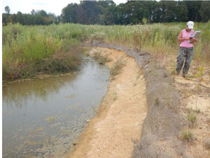
Bare bank Norkett Branch Reach 2 right bank, continuing to erode. 9-21-2015
