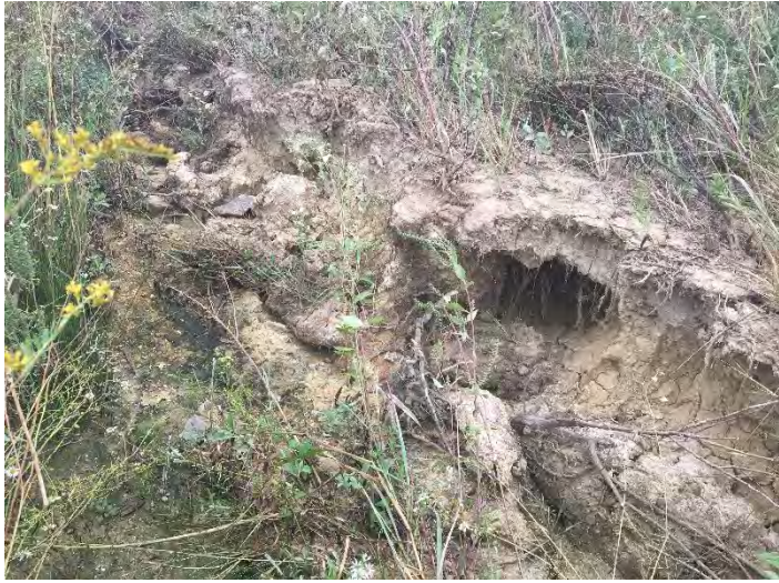
Old Scour: Norkett Branch Station 103+00 – 10/9/2018
