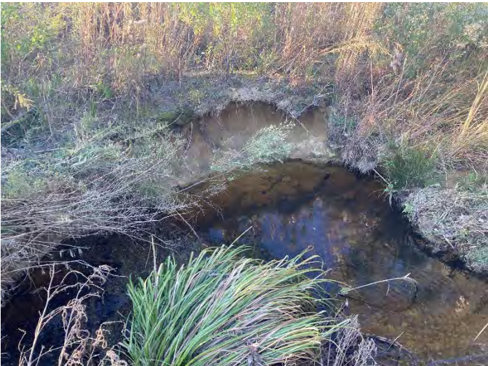
Bank Scour – Norkett Branch Reach 1 11/3/2020
