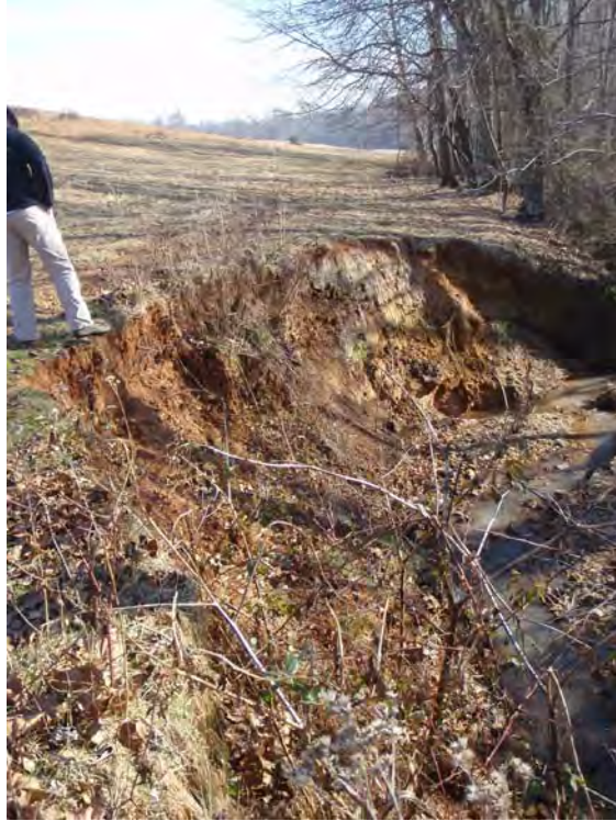
Photo 9 – Bank erosion on Reach 1
