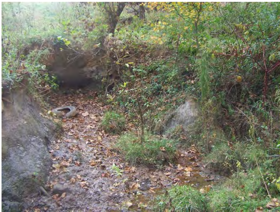
Photo 12 – Headcut on Reach 3
