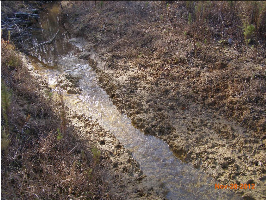
1-S Reach 1 Sta. 305+50 – Riffle Degradation
