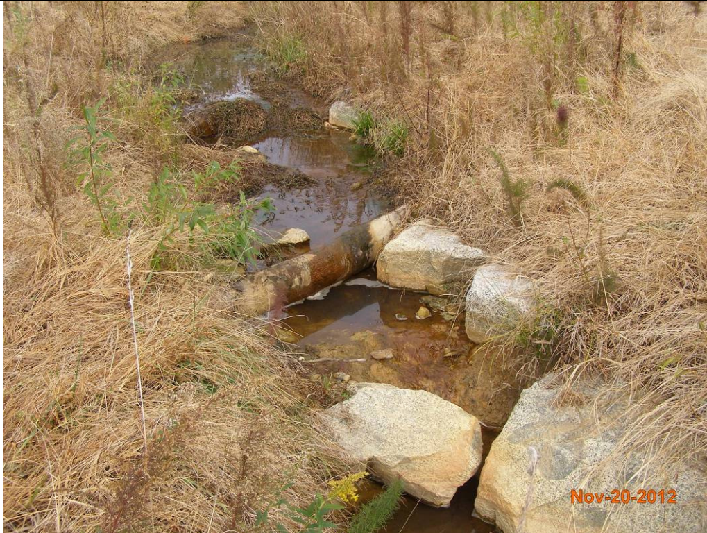
7-S Reach 4 Sta. 102+30 – Stressed Structure
