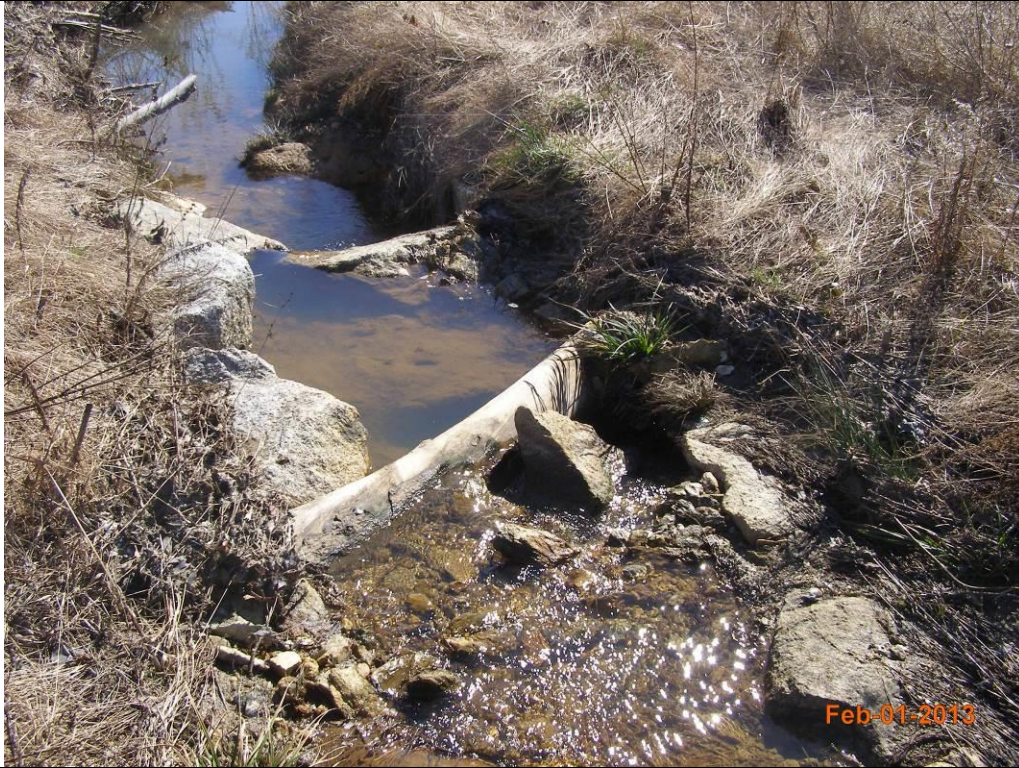
6-S Reach 4 Sta. 102+30 – Stressed Structure
