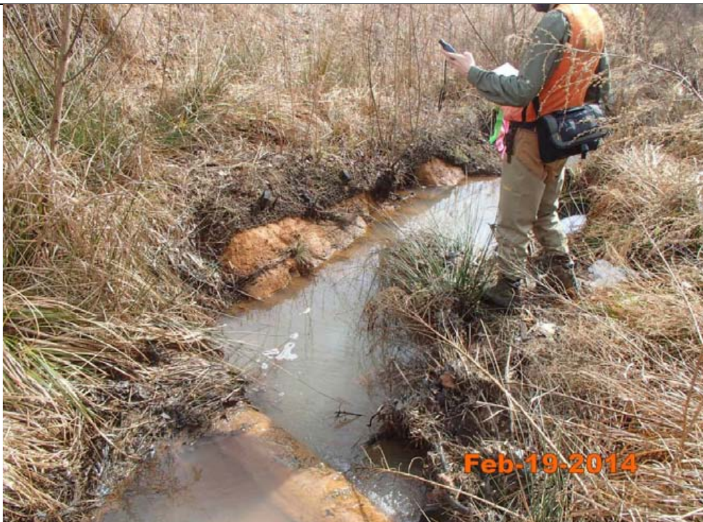
Reach 2 Sta. 107+50—Bed Degradation with Headcut (Looking Downstream)
