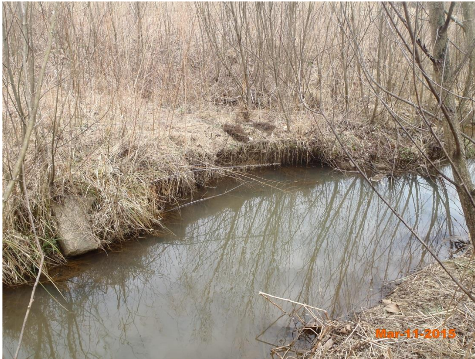
Reach 1 Sta. 321+50—Erosion along Left Descending Bank
