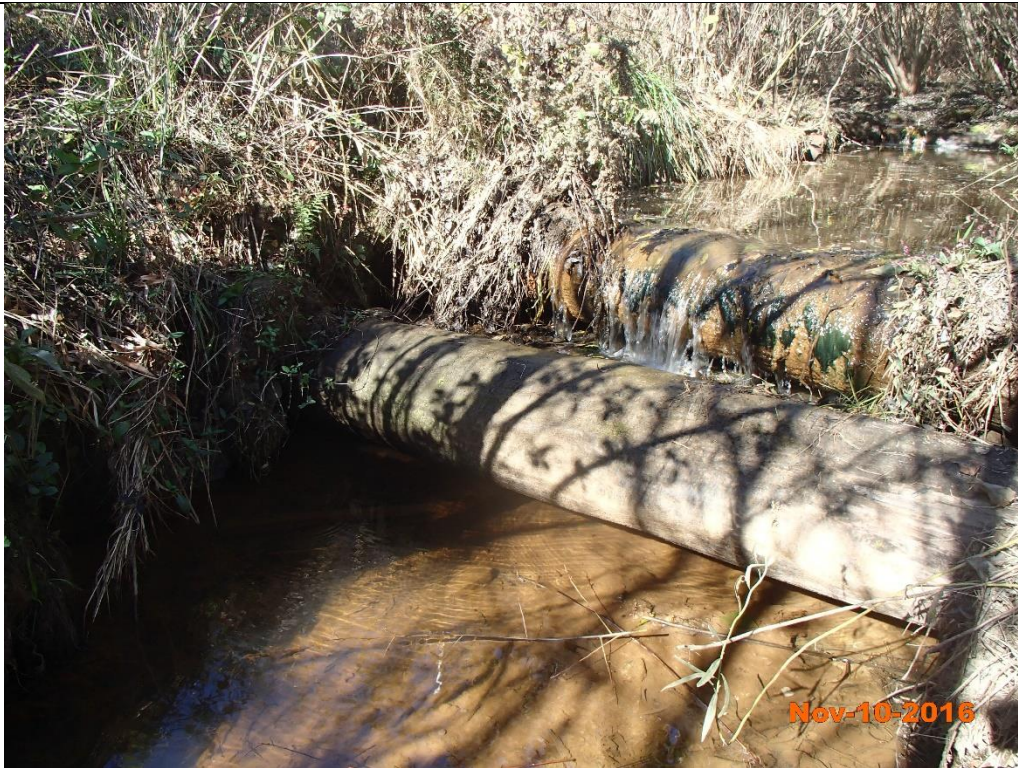
Reach 2 Sta. 106+00– Stressed Structure
