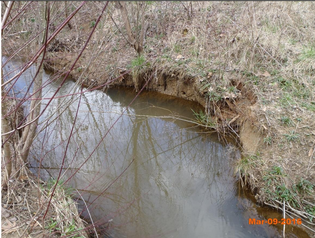
Reach 1 Sta. 316+60 – Bank Erosion
