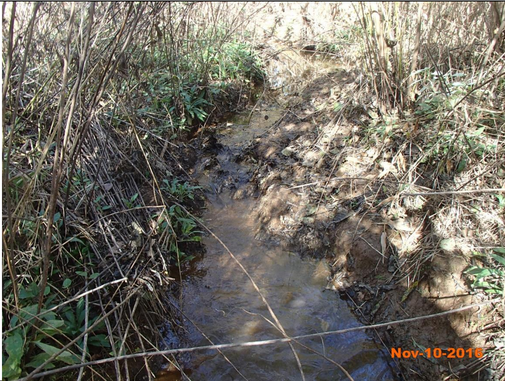
Reach 2 Sta. 110+50 – Headcut/ Bed Degradation
