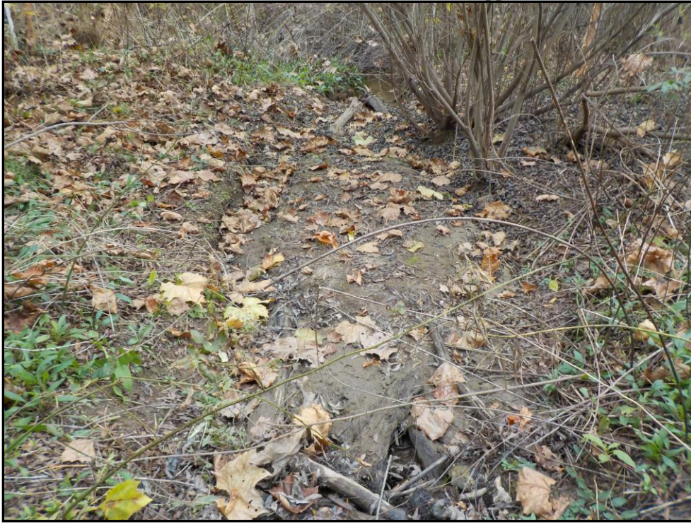
Reach 4 Sta. 101+60 – Bed Aggradation November 14, 2017
