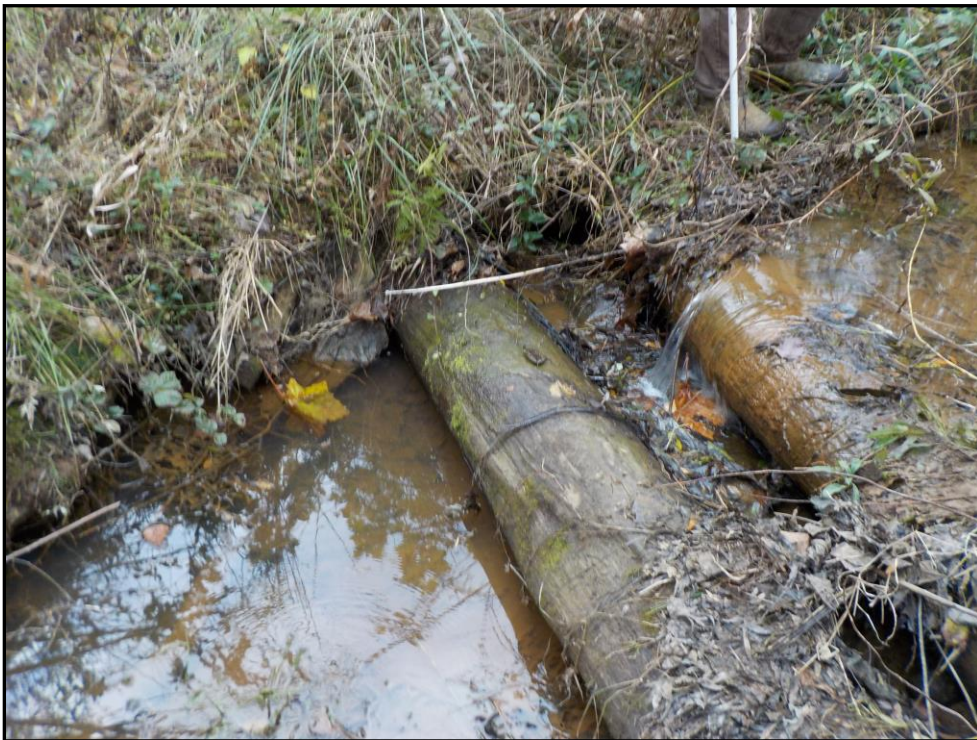
Reach 2 Sta. 106+00 – Stressed Structure November 14, 2017
