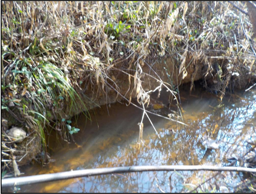
Reach 2 Sta. 118+50 – Bed Degradation & Bank Erosion November 15, 2017
