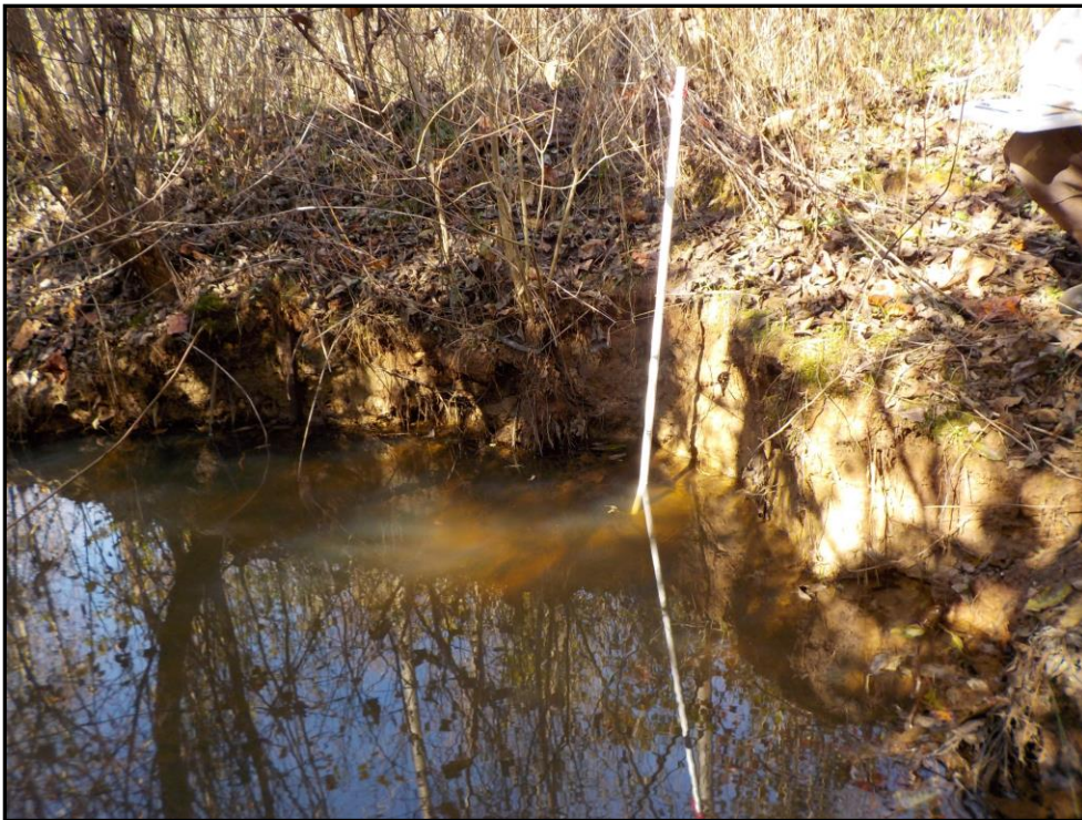
Reach 1 Sta. 318+60 – Bed Degradation & Bank Erosion November 15, 2017
