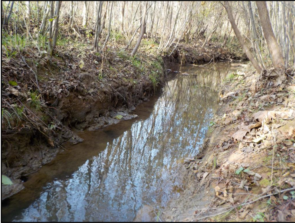
Reach 1 Sta. 314+00 – Bed Degradation November 15, 2017
