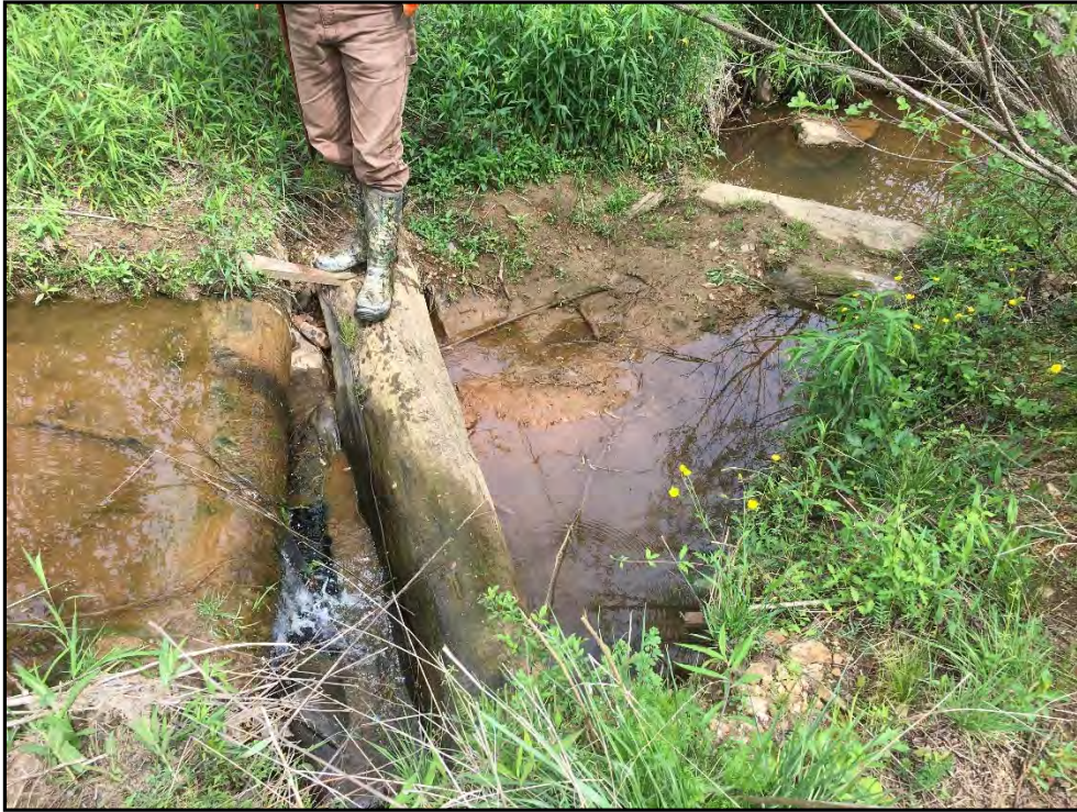
Reach 1 Sta. 106+00 – Stressed Structure (Repaired November 2018)
