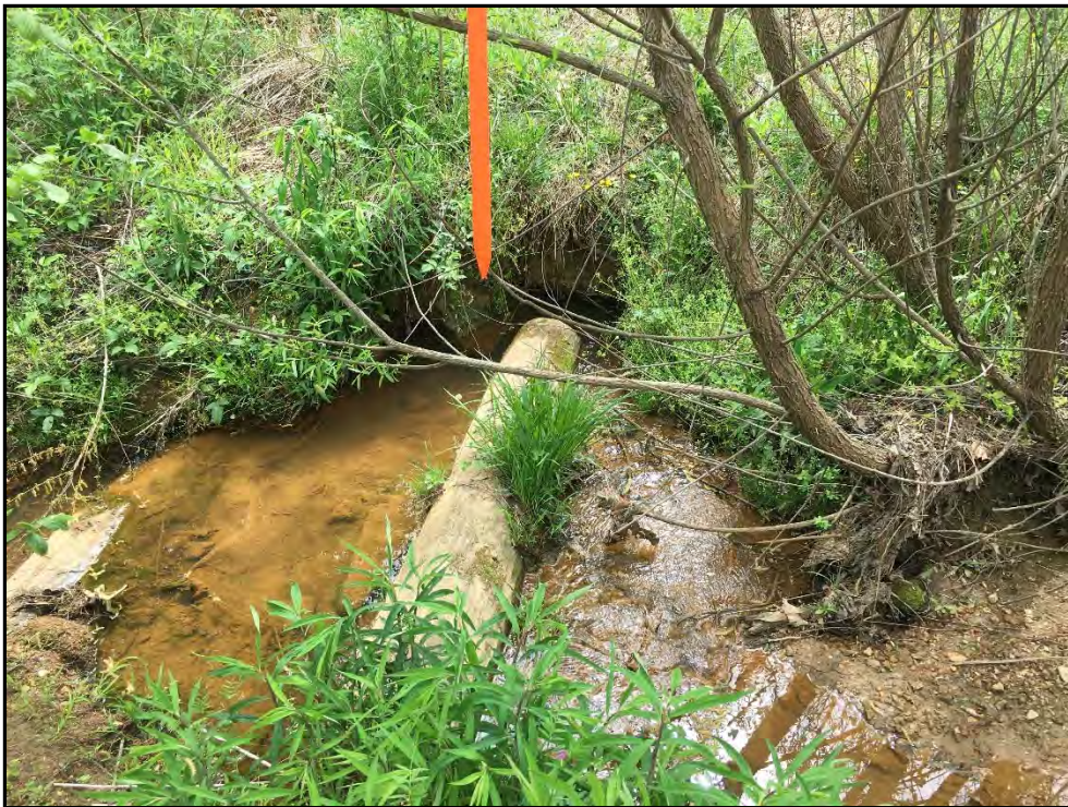
Reach 1 Sta. 106+50 – Stressed Structure (Repaired November 2018)
