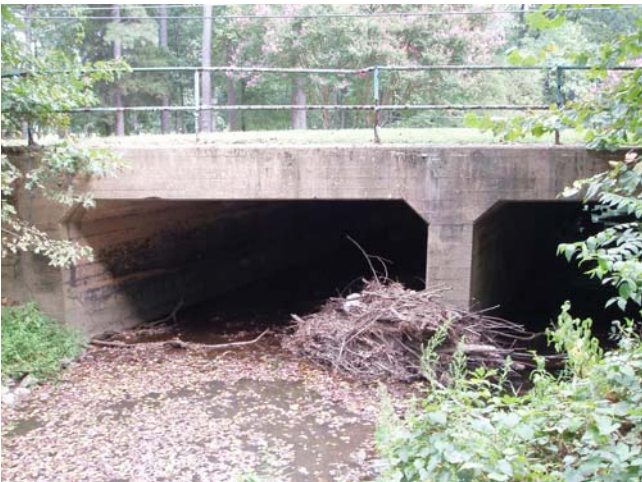
Photo 5. Culverts under Lavender Ave. Debris is gathering against the bridge
