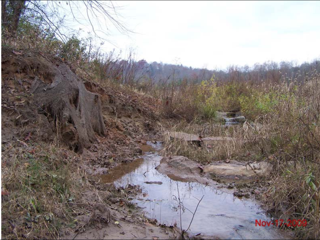
SPA15 UT6 Sta. 610+50 – Bank Erosion and Grade Control Degradation
