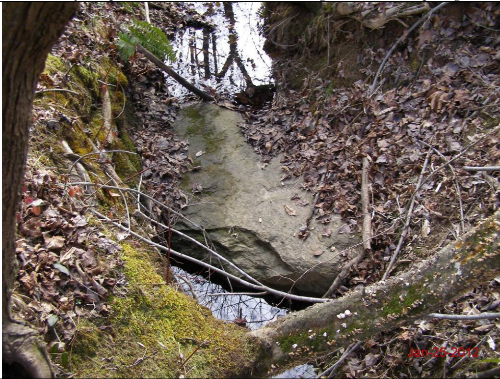
SPA9 UT5 Sta. 515+80 – Grade Control Degradation
