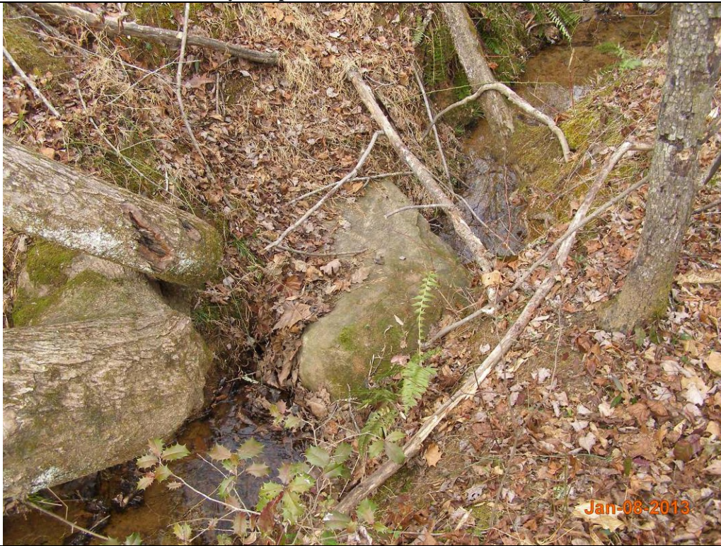
SPA9 UT5 Sta. 515+80 – Grade Control Degradation
