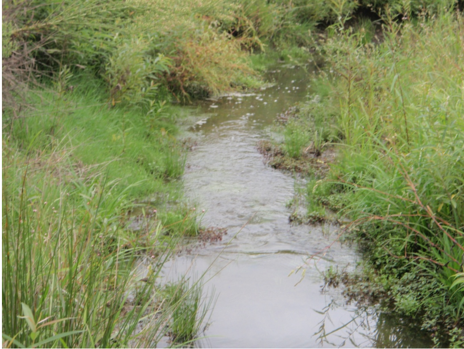
Photo Station S5 – Stream channel looking downstream at cross-section 5 Station 32+71 – Priority 2 (9/23/2011 Year 1)
