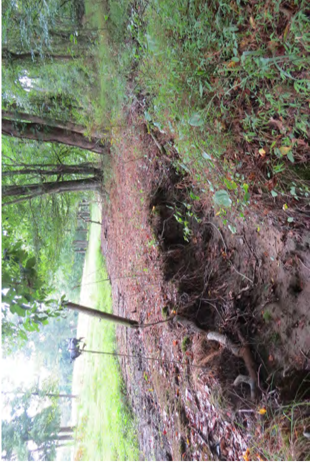
Reach R4 – Eroding banks on meander bend.
