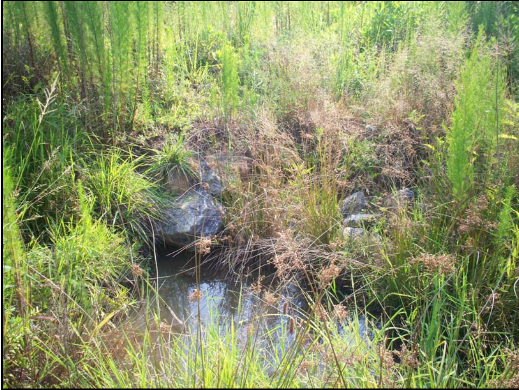
Photo 25. SPA 5. Minor left bank erosion occurring behind rip rap STA 20+25.
