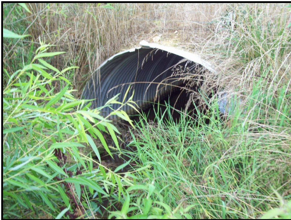
SPA2. Displaced RCV at station 8+65.
