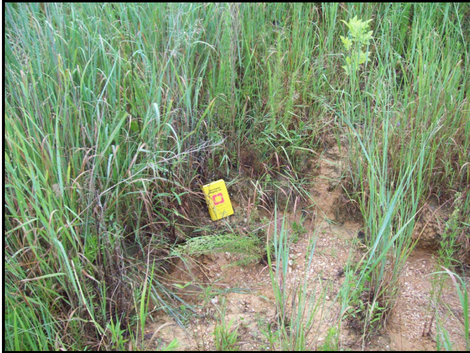
SPA5. Left bank erosion, head cut and rills forming at station 31+85.
