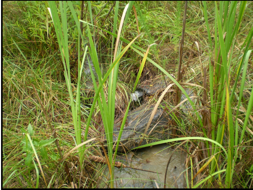
SPA 3 – Header rock on cross weir displaced, UT1 Sta. 28+00.
