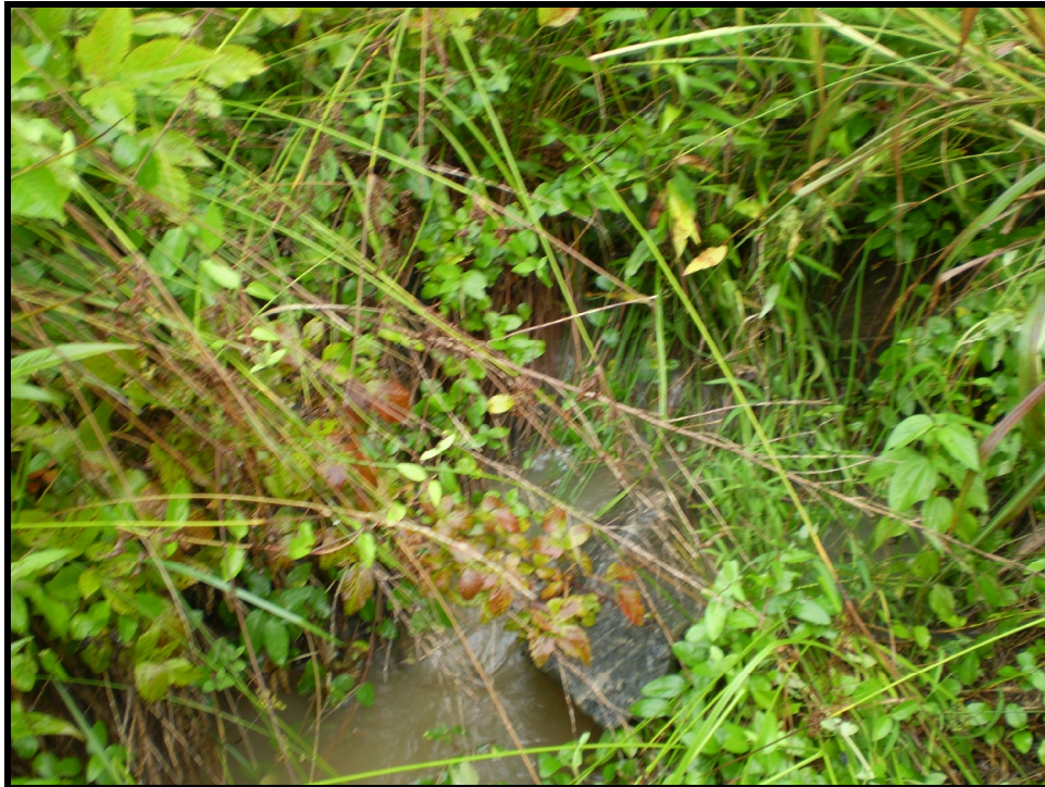
SPA 4 – Rock on cross weir displaced, UT1 Sta. 32+02.
