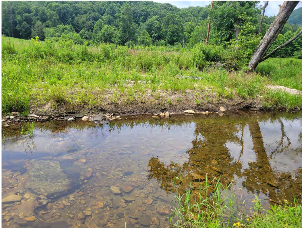
P1: Bank erosion between Station 10+00 and 10+50
