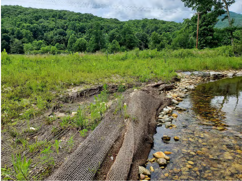
P3: Bank erosion slightly upstream from P2
