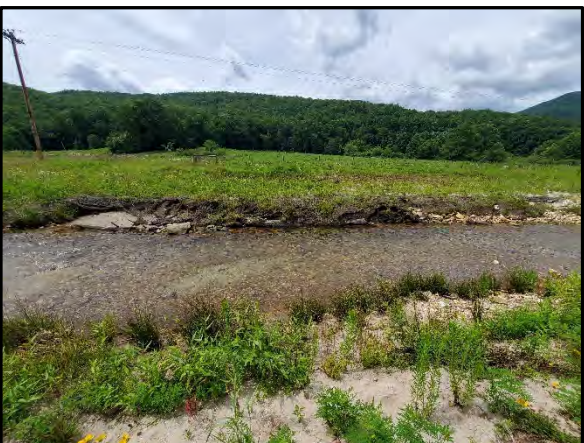
3.47 Bank Erosion between STA 13+90 and STA 14+50 WFFBR, 8/15/2022
