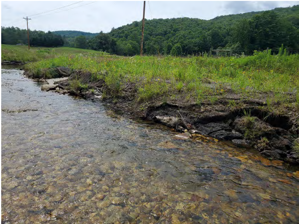
P4: Looking downstream at eroded right bank by Station 14+00
