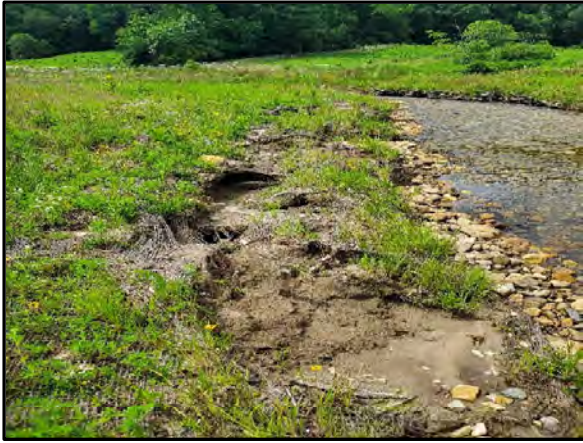
3.49 Bank erosion between STA 16+10 and STA 16+75 WFFBR, 8/15/2022
