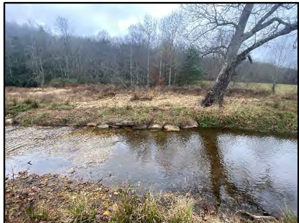
3.54 Toe erosion repair using boulder toe and sod mats from STA 25+15 to STA 25+50 WFFBR, 11/11/2022
