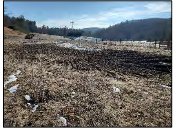
3.38 Floodplain scour repair at right overbank near STA 12+50, 2/1/2022
