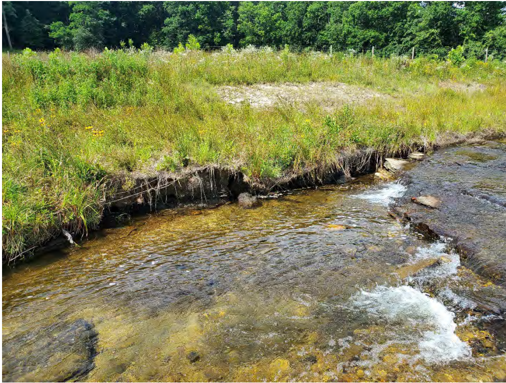
P9: Bank looking upstream at bank erosion on right bank near Station 22+50
