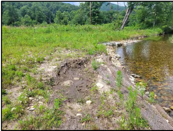
3.45 Bank erosion at STA 10+70 to 11+25 WFFBR, 8/15/2022
