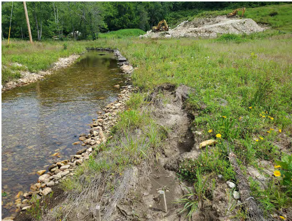
P8: Looking upstream at scour/bank erosion shown in P7
