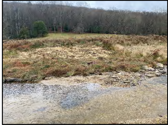
3.52 Toe erosion repair using boulder toe and sod mats from STA 22+35 to STA 22+95 WFFBR, 11/11/2022
