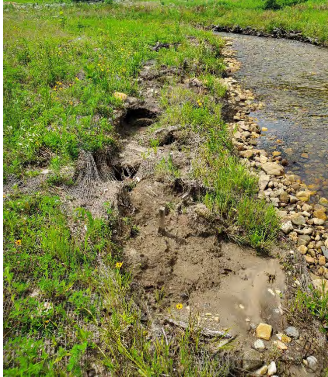
P7: Looking downstream at scour/bank erosion on left bank near Station 16+50
