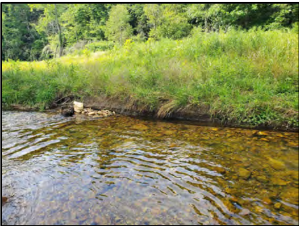
3.53 Toe erosion between STA 25+15 and STA 25+50 WFFBR, 8/15/2022
