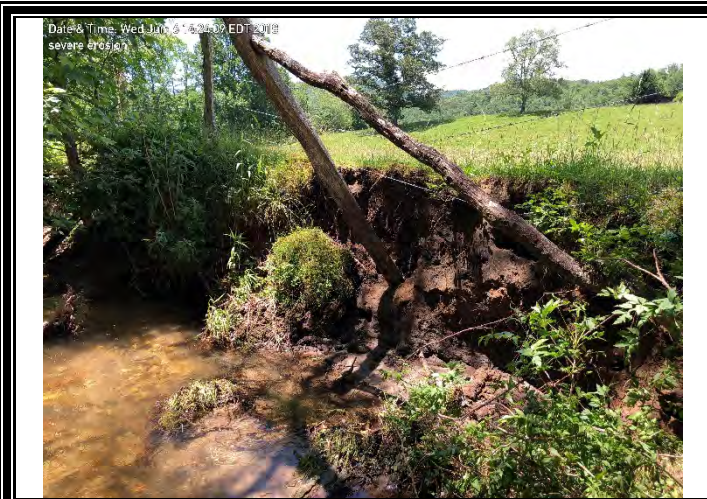
Area of severe erosion along enhancement section of WFFBR
