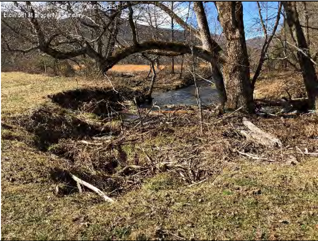
Eroding bank along WFFBR near beginning of project
