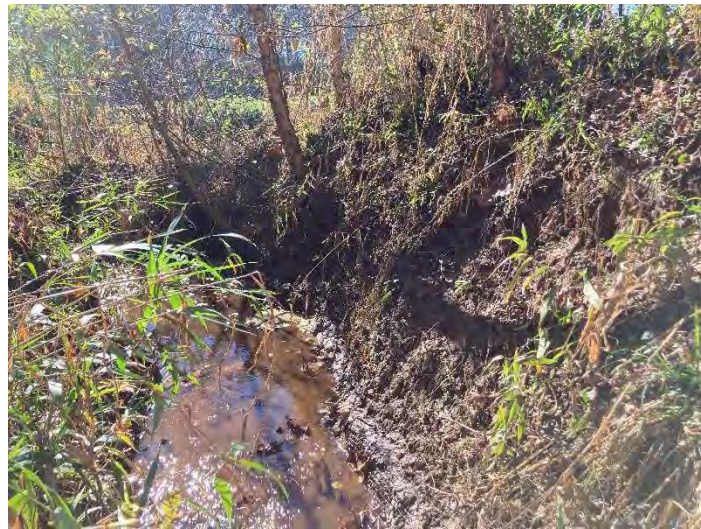
HC1 Reach 2, station 117+50 to 117+79 – Bank scour (11/8/2022)
