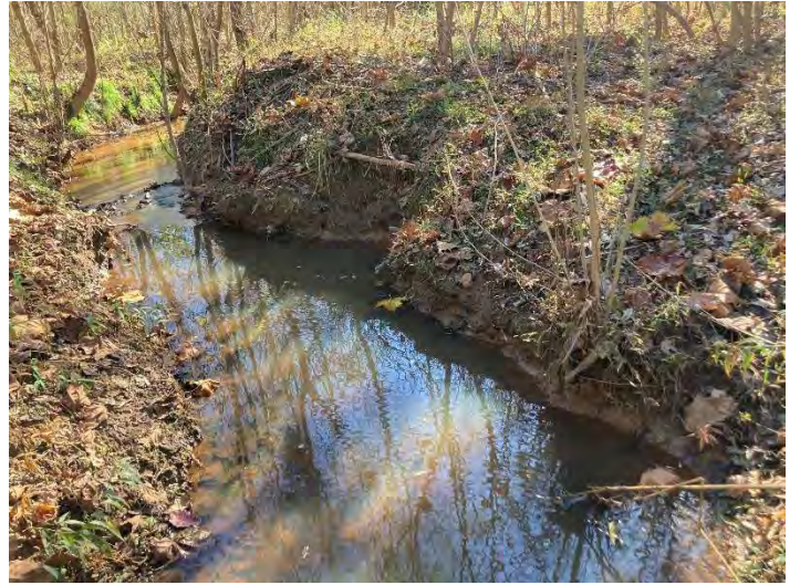
HC1 Reach 2, station 116+40 – Bank scour (11/8/2022)
