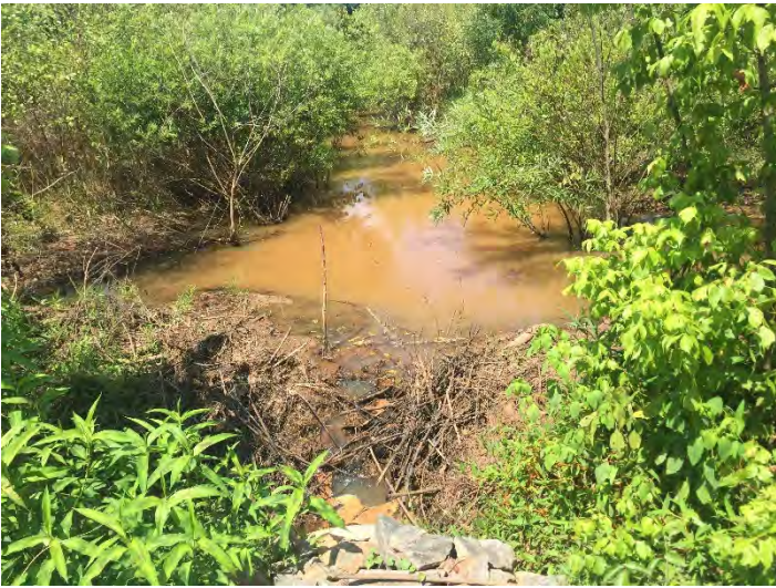
Beaver Dam above Culvert (7/2/2020)
