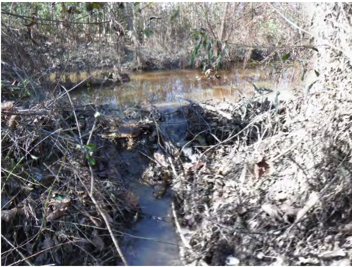
Re-built Beaver Dam below Culvert at XS7 (11/5/2020)
