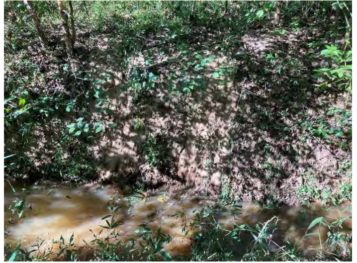
Vertical left bank on HC1 Reach 2; extends from station 117+50 to station 117+79 (10/18/2021)
