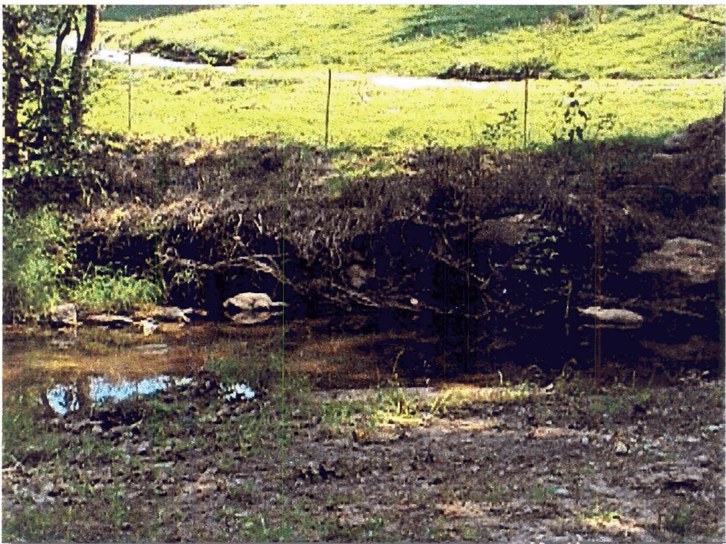
Top photo shows concave side of meander after construction and installation of erosion control material and root-wads. Bottom photo shows flood-plain bench matching the upstream bank with cover crop vegetation, trees and fence 3 months after construction.
