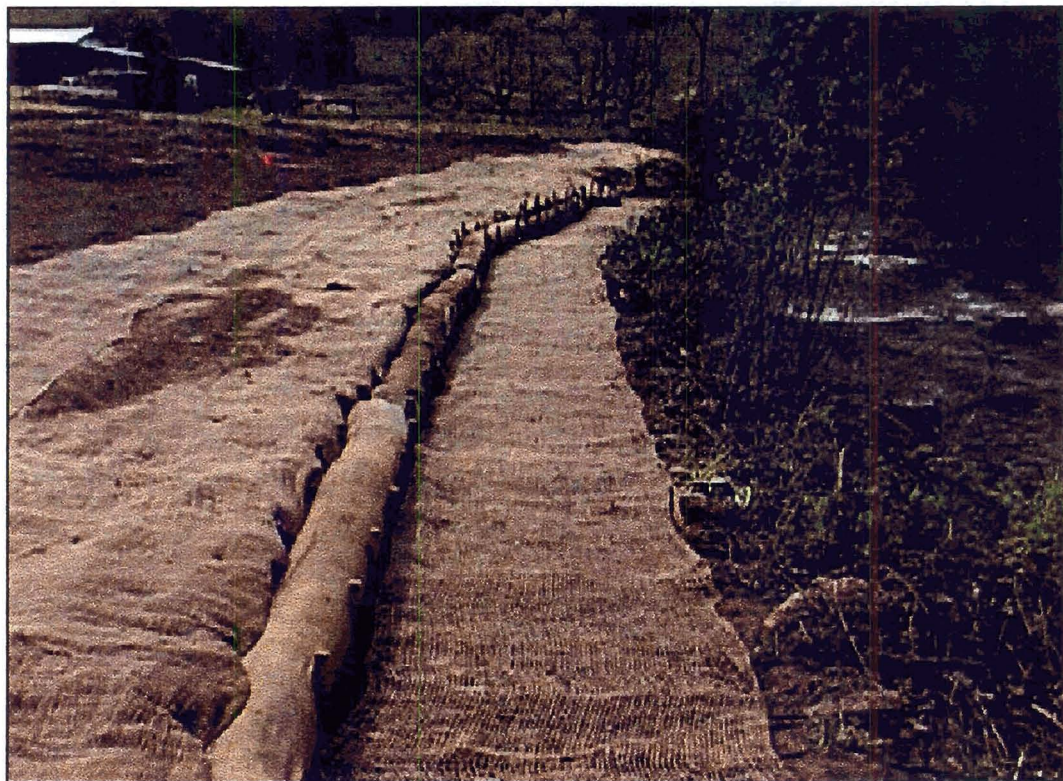
Top photo shows typical condition of stream banks at this site prior to construction. Bottom photo shows typical construction methods used to address vertical bank conditions. Banks are sloped, fertilized, limed, seeded and erosion matting installed. Coir logs are pinned at the bankfull elevation and trees are planted behind this log to provide long-term stability.
