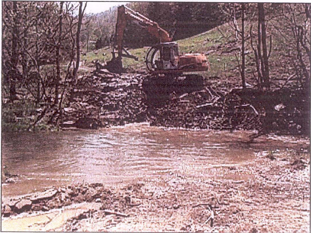
Big bend below driveway bridge. Top photo shows the existing conditions with erosion and auto parts as stabilizing material. Bottom photo shows removing auto parts and trash and installing root-wads and creating floodplain to match existing bench upstream.
