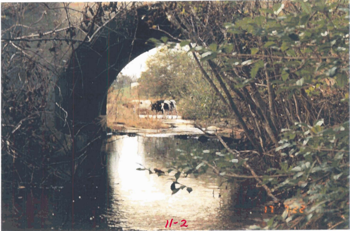
#3 – Cattle crossing just downstream of SR 1605. Looking downstream through culvert under SR 1605.
