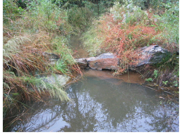
Issue Photo 1. Piping through structure Station: Just upstream of Area 2.
