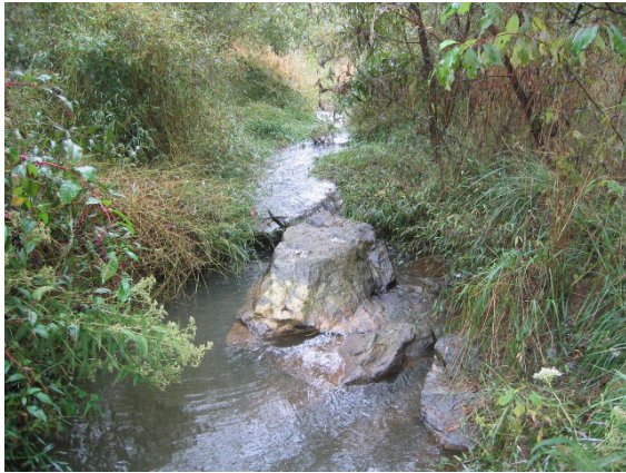
Issue Photo 2. Slumped cross vane arm. Located just upstream of Paul Payne Road culvert. A cross vane 20 feet downstream is holding grade.
