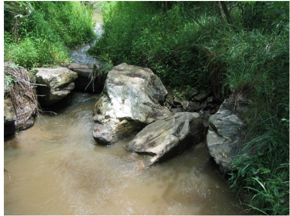
Issue Photo 2. Slumped cross vane arm. Located just upstream of Paul Payne Road culvert. A cross vane 20 feet downstream is holding grade.
