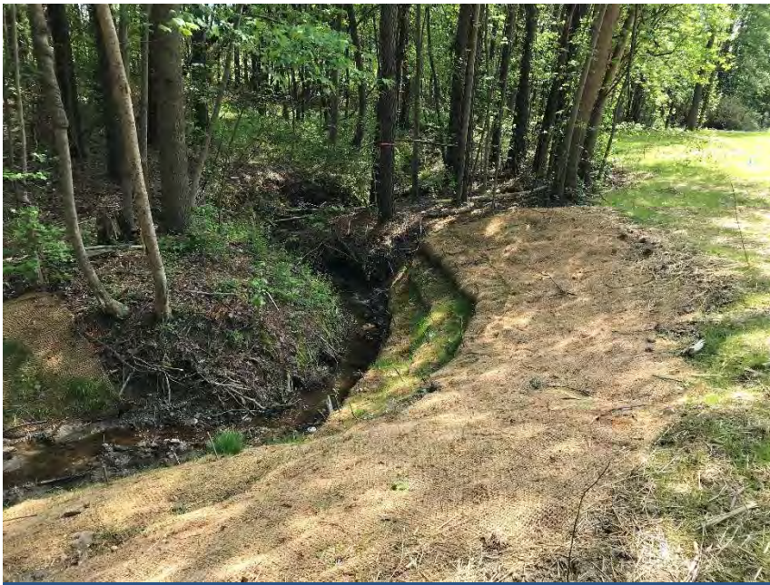
PS-2, R2, facing downstream, Sta 21+50, April 27, 2018 (MY-00)
