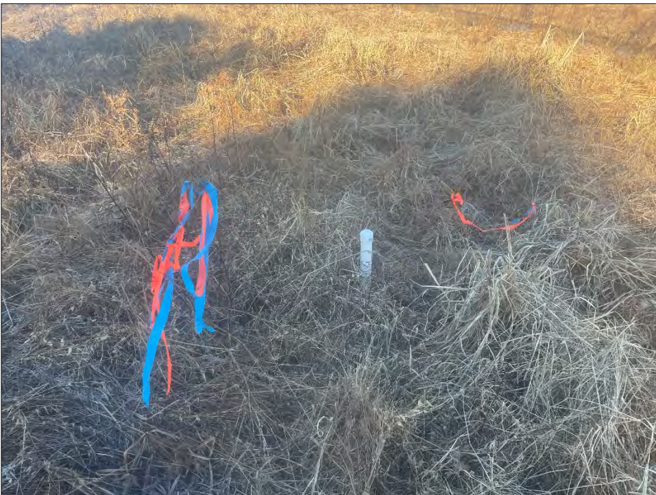
Groundwater gauge installed - 01/11/2022
