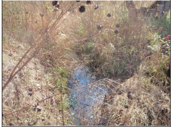
Photo Point 123 – Log Weir, UT6
