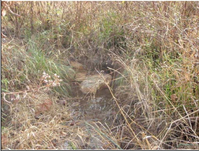
Photo Point 122 – Log Weir, UT6
