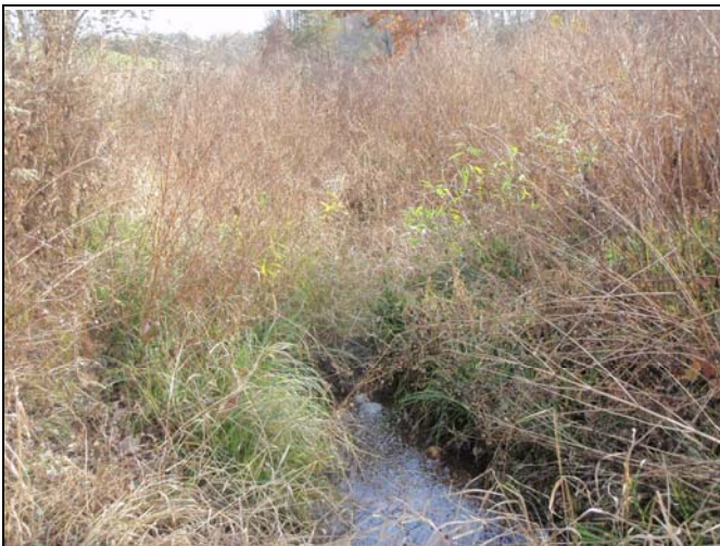
Photo Point 126 – Log Weir, UT6
