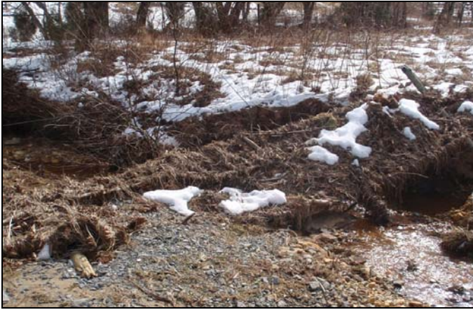
BEFORE: UT1_R3 stream crossing after storm damage near station 57+00
