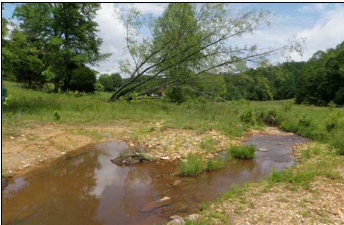
BEFORE: Looking downstream at left bank erosion from January 2010 storm damage
