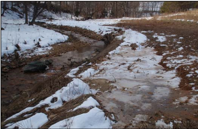
AFTER: Repaired left bank and installed geolift at UT1_R4 station 67+00, view is upstream
