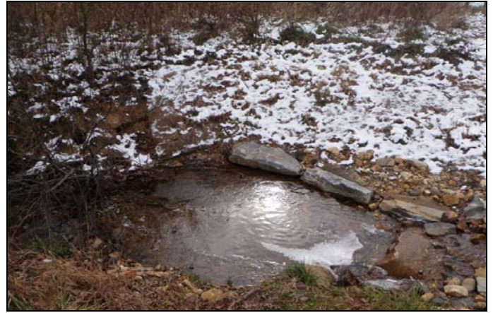
AFTER: UT1_R3 repaired stream crossing by adding Class I/B stone and installed a grade control J-Hook
