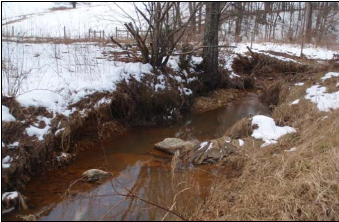
BEFORE: Observed right bank erosion and structure failure along UT1_R3 near station 57+75
