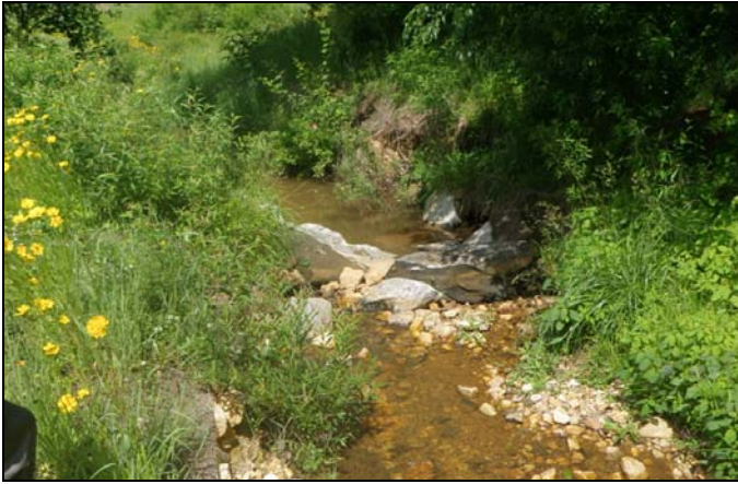
BEFORE: Repaired cross vane piping and right bank erosion along UT5_R1 near station 18+25
