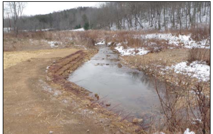
AFTER: Repaired left bank and installed geolift at UT1_R4 near station 74+00, view is downstream
