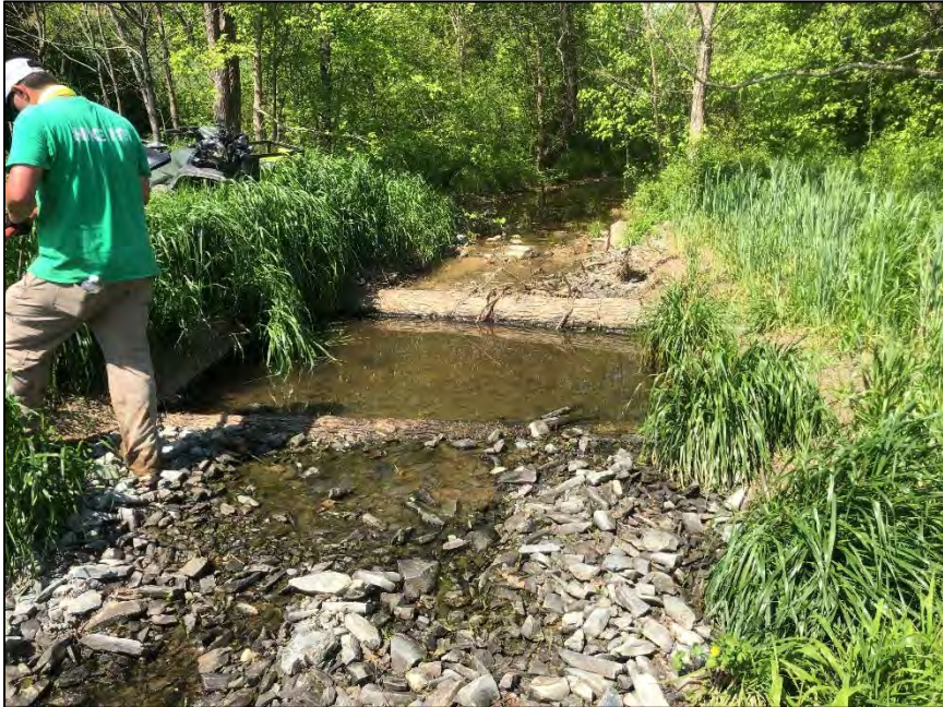
Newly replaced log sill at the top of the reach (Area 1 from AMP) looking upstream
