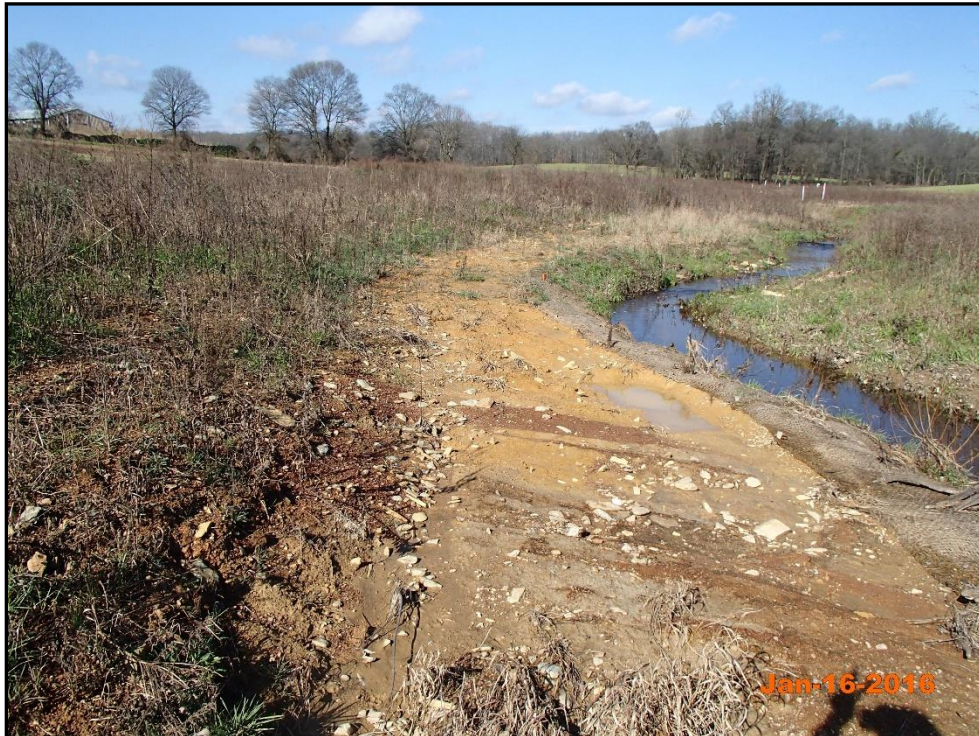
Project Reach UT1-3 – Bare Area 29+00 Right Descending Bank
