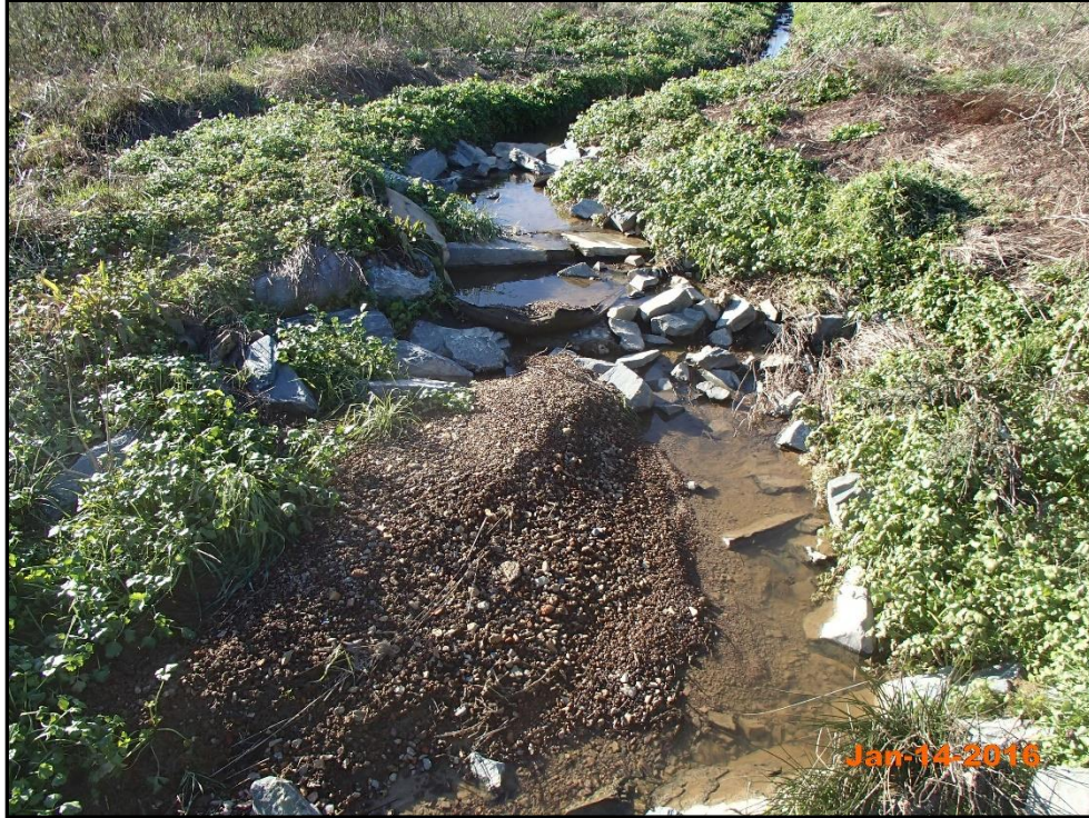
Project Reach UT2-A – Stressed Structure 3+75 Left Descending Bank
