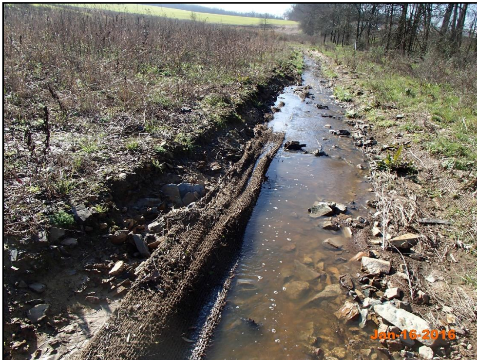
Project Reach UT1-B – Bank Erosion 7+25 Left Descending Bank
