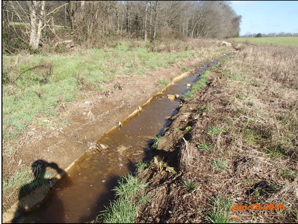
Project Reach UT1-B – Degradation 8+25 Left Descending Bank
