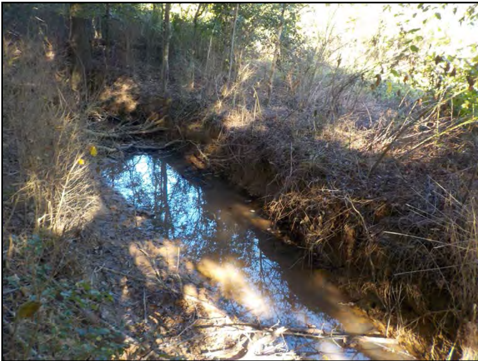
UT1-1 – Left and Right Bank Erosion
