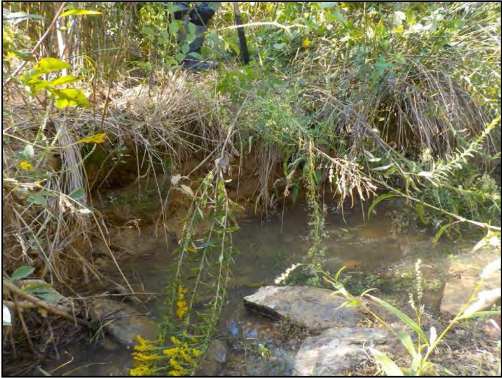
UT1-C – Right Bank Erosion
