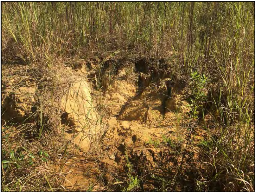
UT1-2 – Left Bank Erosion
